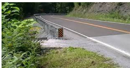
Example of high friction surface treatment (left) [FHWA].
